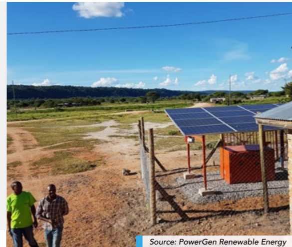
Source: PowerGen Renewable Energy
