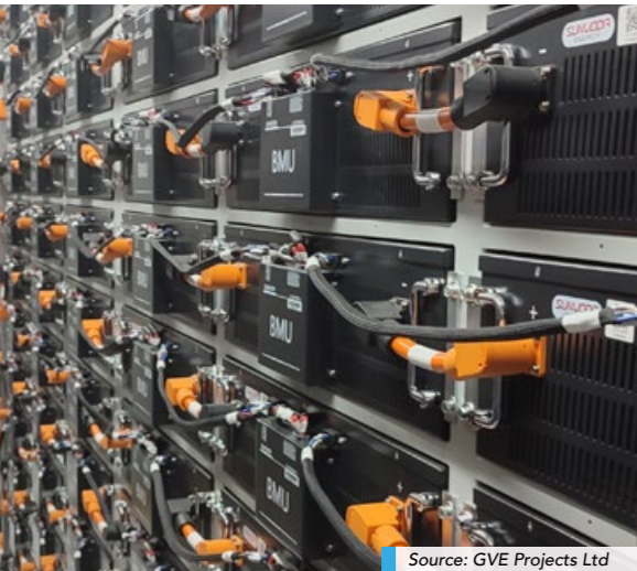
Source: GVE Projects Ltd
