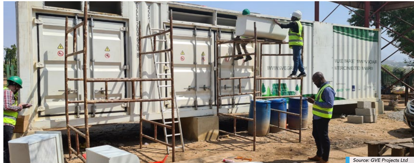
Source: GVE Projects Ltd
