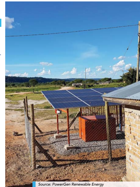
Source: PowerGen Renewable Energy
